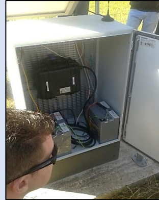
Recording equipment and back-up electricity supply for a Gulf of Corinth seismometer
