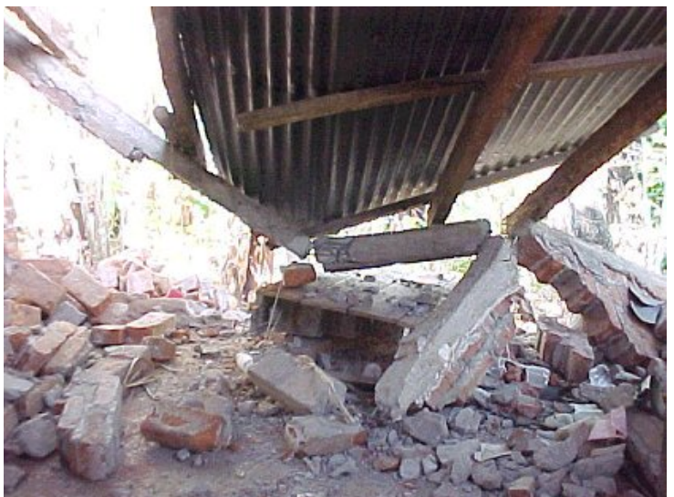
Figure 5.1: A school in San Salvador destroyed by an earthquake.
