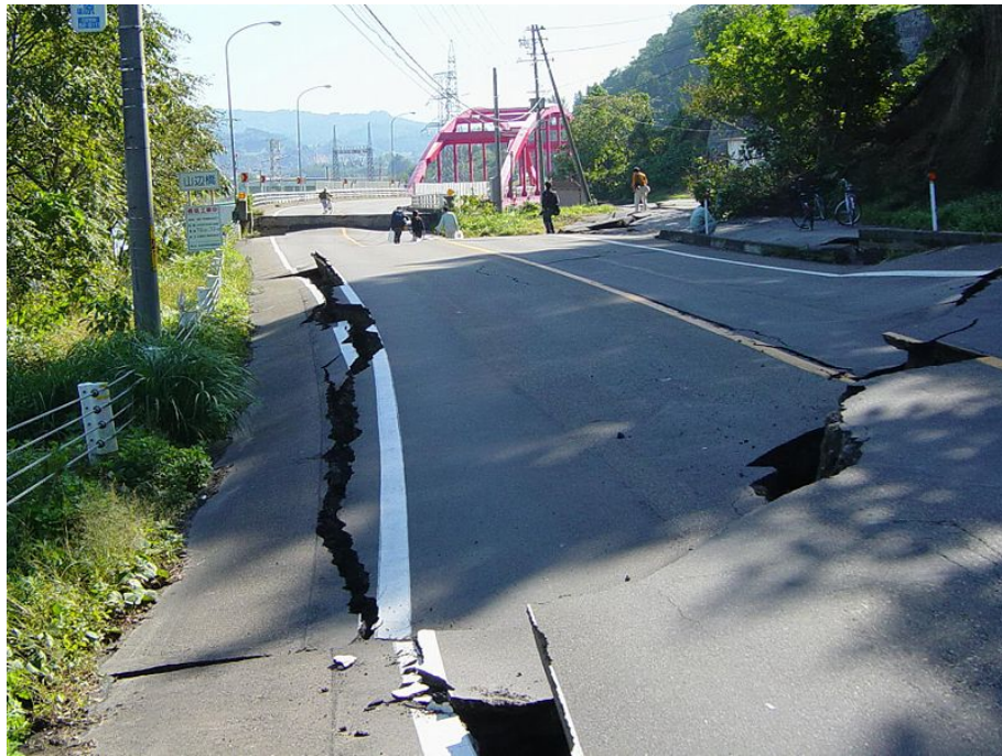
Figure 5.3: Earthquake damage in Japan - Chuetsu earthquake, 2004.
