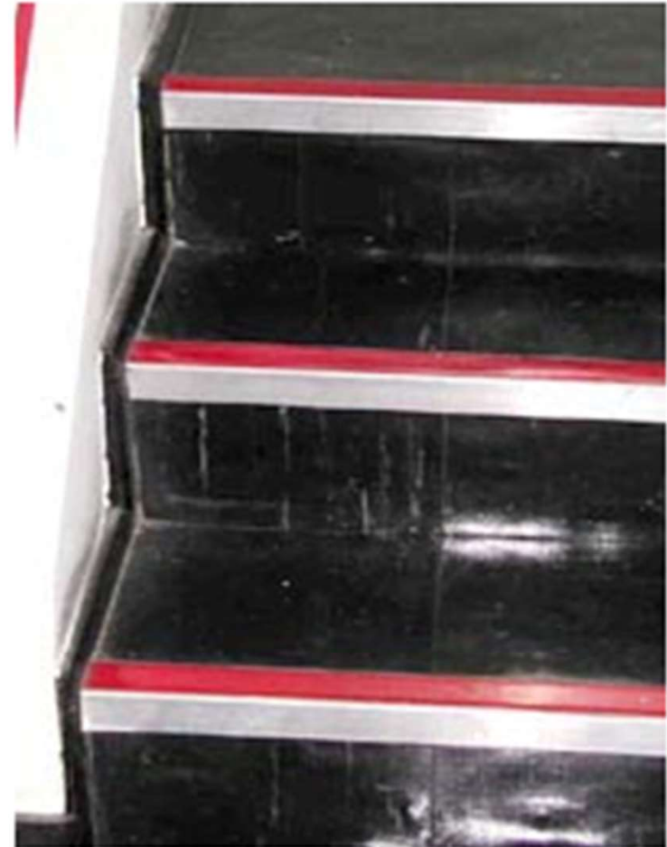
Fig. 2-5 Rubber strips on staircases help to increase friction and prevent slippery.
