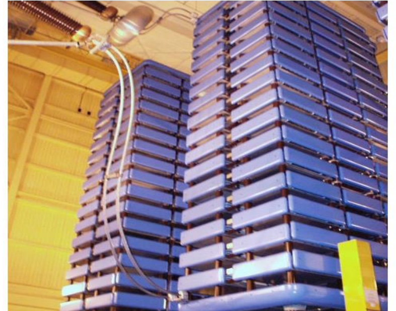
Manitoba Hydro Thyristor Valves
