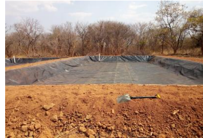
Lined earthen diversion pond constructed by above ground embankments (dykes), the pond will be supplied by borehole water and is completely drainable
