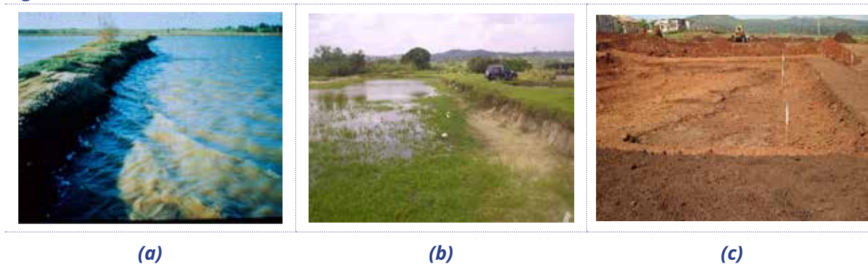
Figure 17: Erosion of Pond Walls
